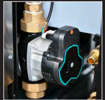
Circuit pump of heating
